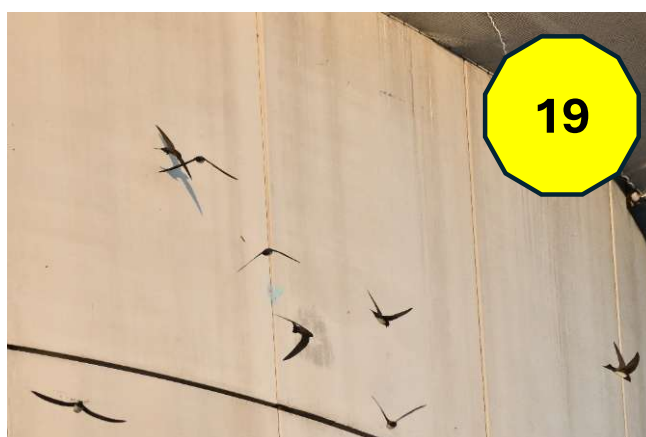
Alpine swifts crowding in front of a horizontal expansion joint. Photo Milo Manica
