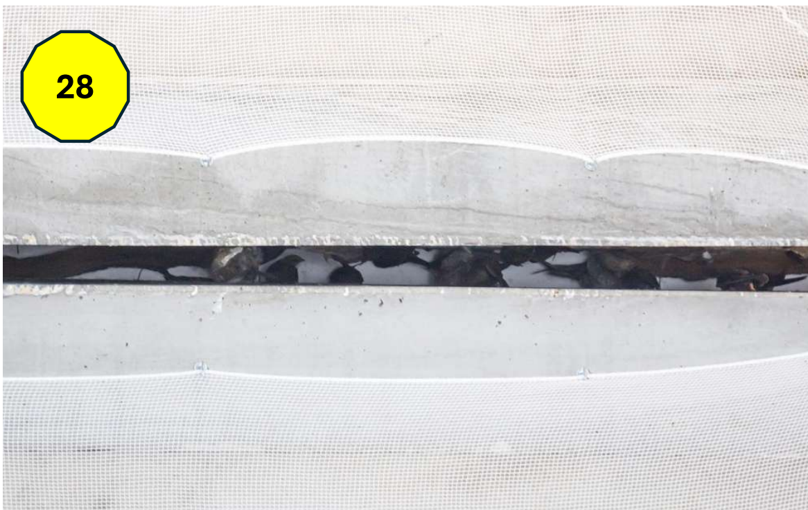
In this image the edges of the two nets that should have prevented access to the crack are evident but leave it free, and the swifts have occupied it. photo Gaspare Fiorentino
